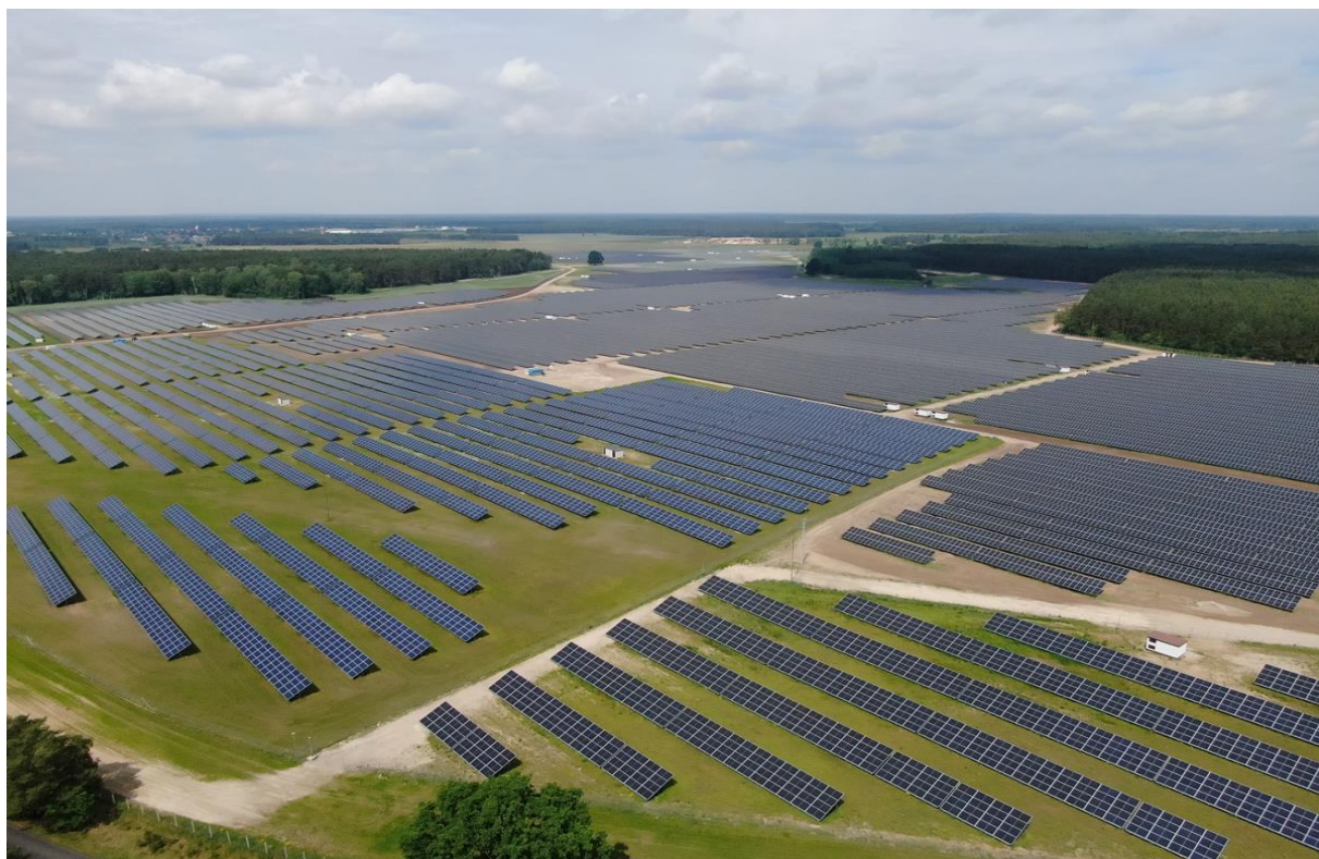
Wielbark photovoltaic Farm
