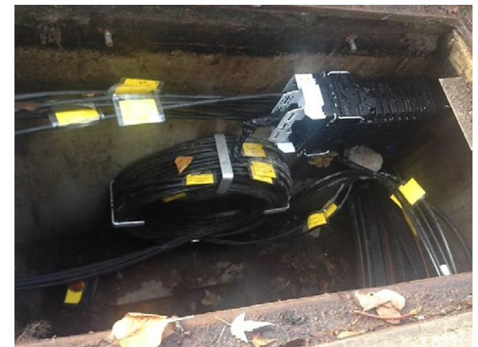
Fiber optic access network
