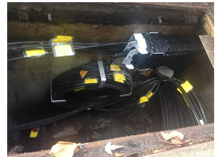
Fiber optic access network
