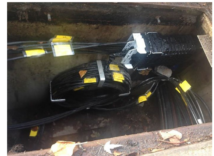
Fiber optic access network
