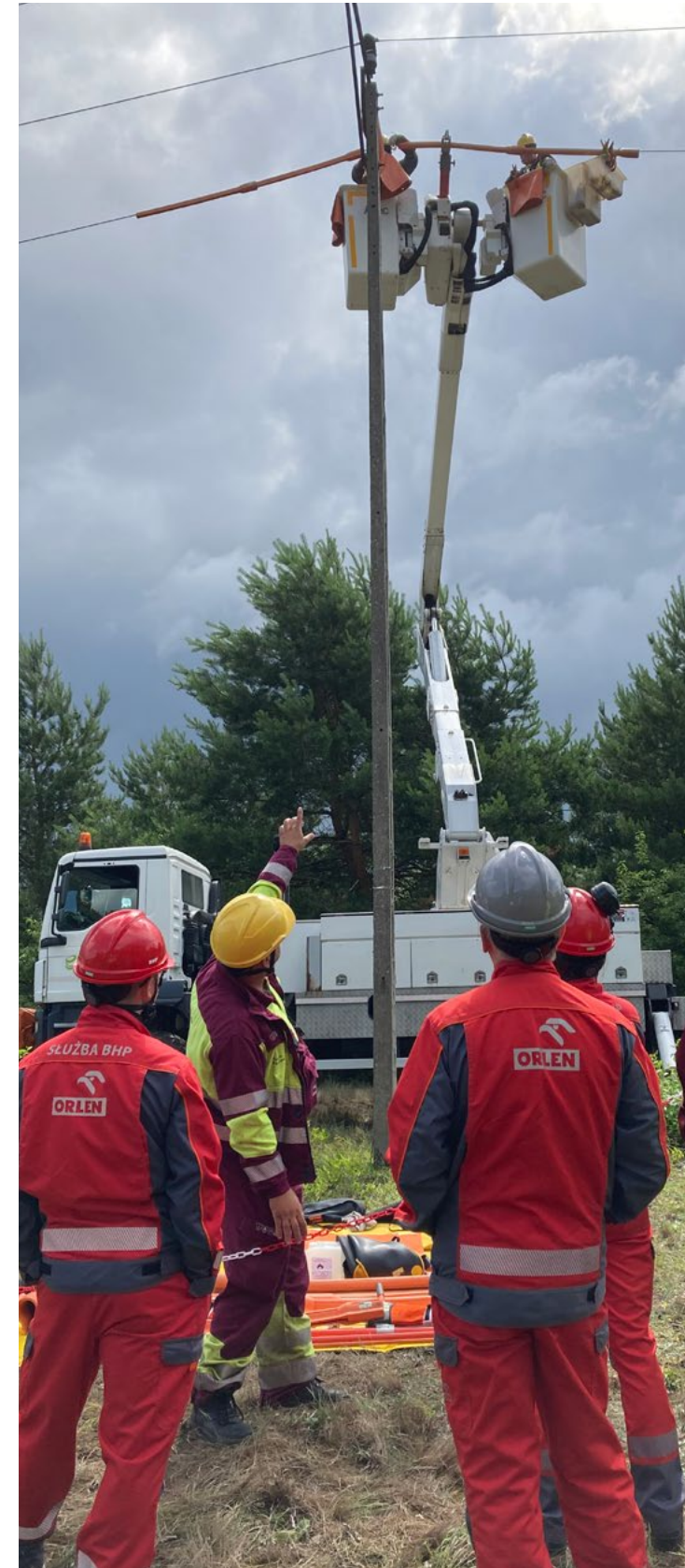
Advisory visit of OHS Services of ORLEN Capital Group companies during works in live technology on a 15 kV line carried out by Energa-Operator Branch in Toruń.
